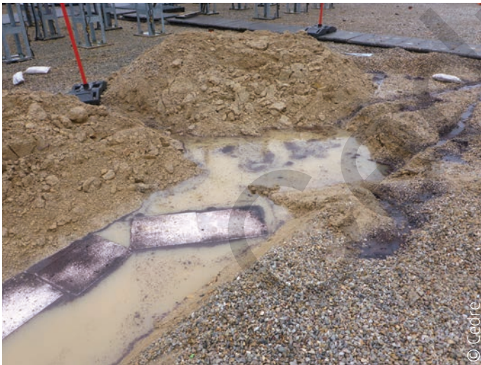
Sorbent pads and peat in a trench to contain an oil spill
