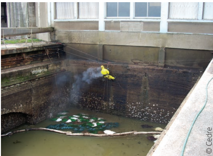
A rope access technician cleaning walls, recovery of washing effluents with sorbents
