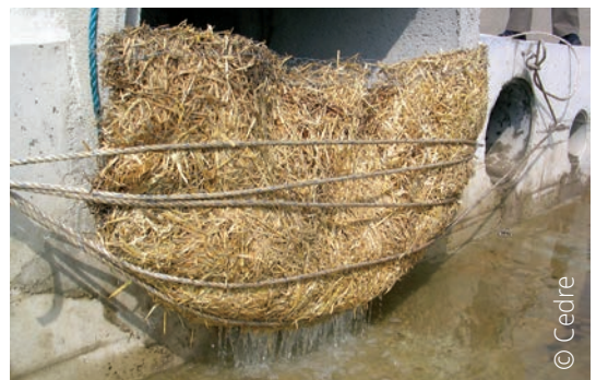
A filter cartridge installed at an outfall
