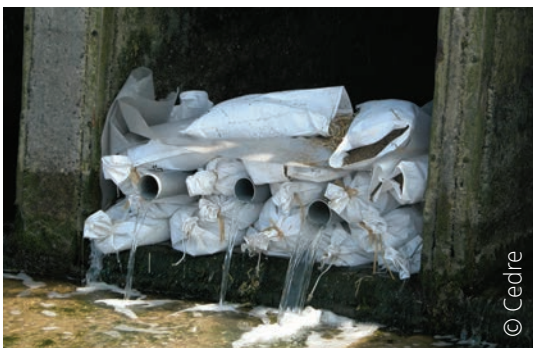
Containment and water level management with a dam made of bags of rubble
