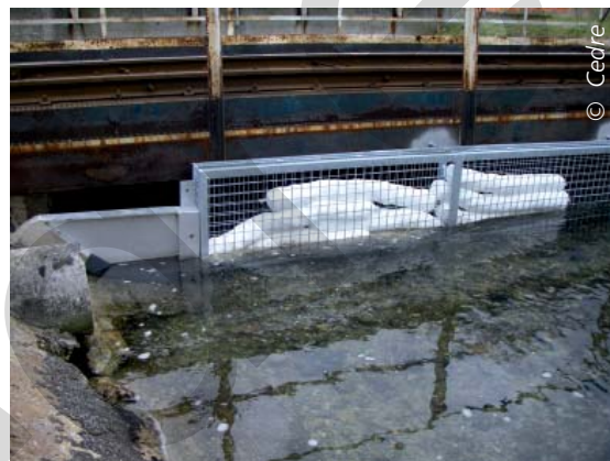
Filtration system for industrial discharge
