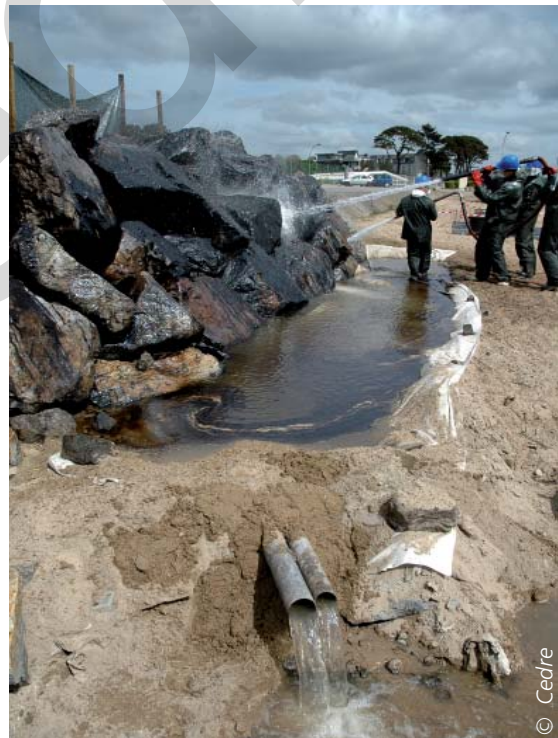
Retention trench for washing effluents, protected by geotextile
