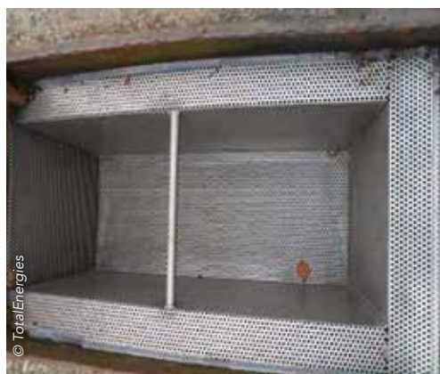
Figure 21. Example of a device installed in a drain.
