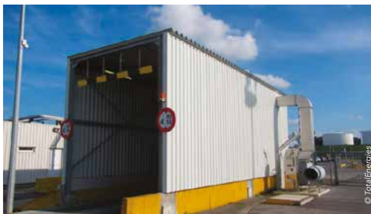
Figure 22. Example of a blower unit for cleaning trucks.
