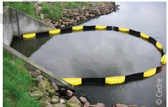
A permanent boom installed at an outfall
