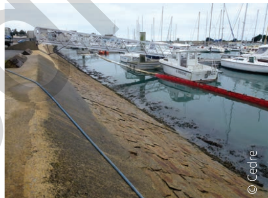
Oiled quay and containment using booms
